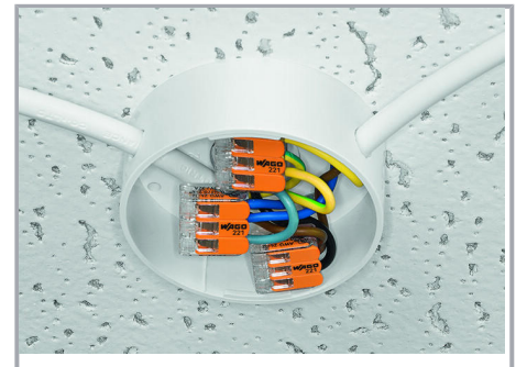
Lighting distribution in ceiling canopy
